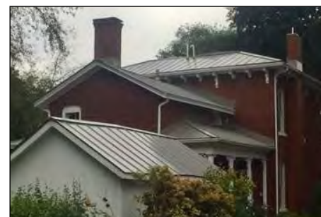
"After." Completed sections of the house as in the "During" image, taken at ground level.
