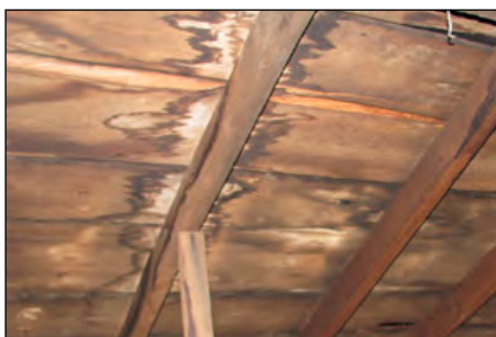
"Before." Water stains are evidence of the roof leaks in the attic.
