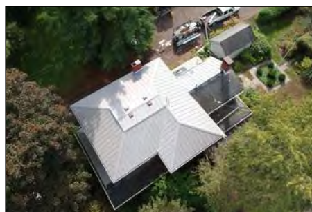
"During." Photo taken by a drone showing the completed upper level roof and a partially completed south-facing roof over the kitchen.
